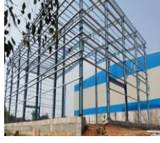
Infra building, Raipur
